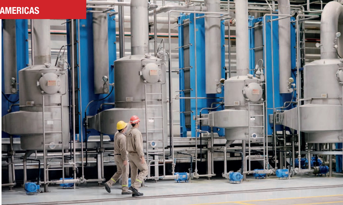
Citrusvil's Plant in Ceivil Pozo, Tucumán, Argentina
